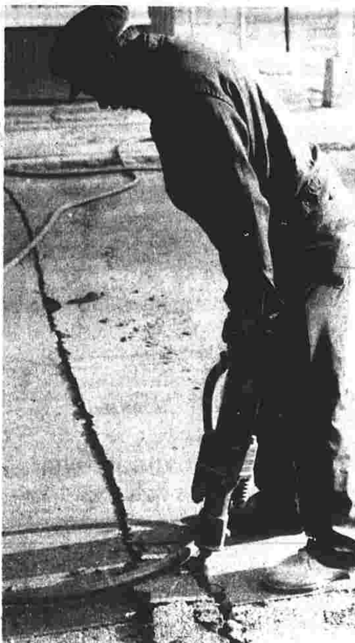
Road worker Joe Parker uses a jackhammer to tear into Bissell Street near its intersection with Spruce Street. Parker is an employee of the Ameron Corp. of New Jersey which is under contract with the town to reline about 9 miles of water mains. (Herald photo by Pinto)
